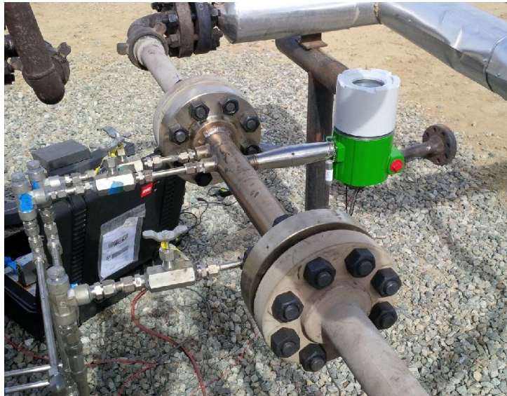
Fig 1. 3" Saturated Steam VorCone Meter at a Heavy Oil Field Injection Point.
