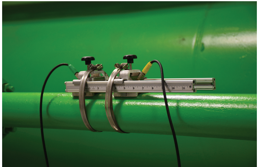
▲ Figure 2: Clamp-on ultrasonic transducers mounted to water line.
